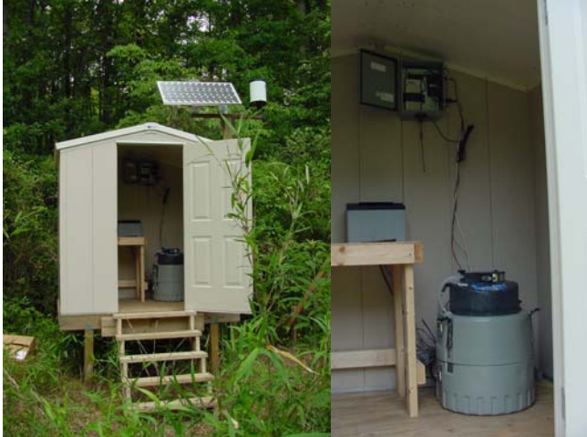
Figure 2. Sampling shed showing ISCO sampler, solar panel and wireless communication device.
